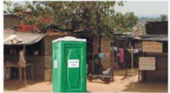
On site temporary sanitation
